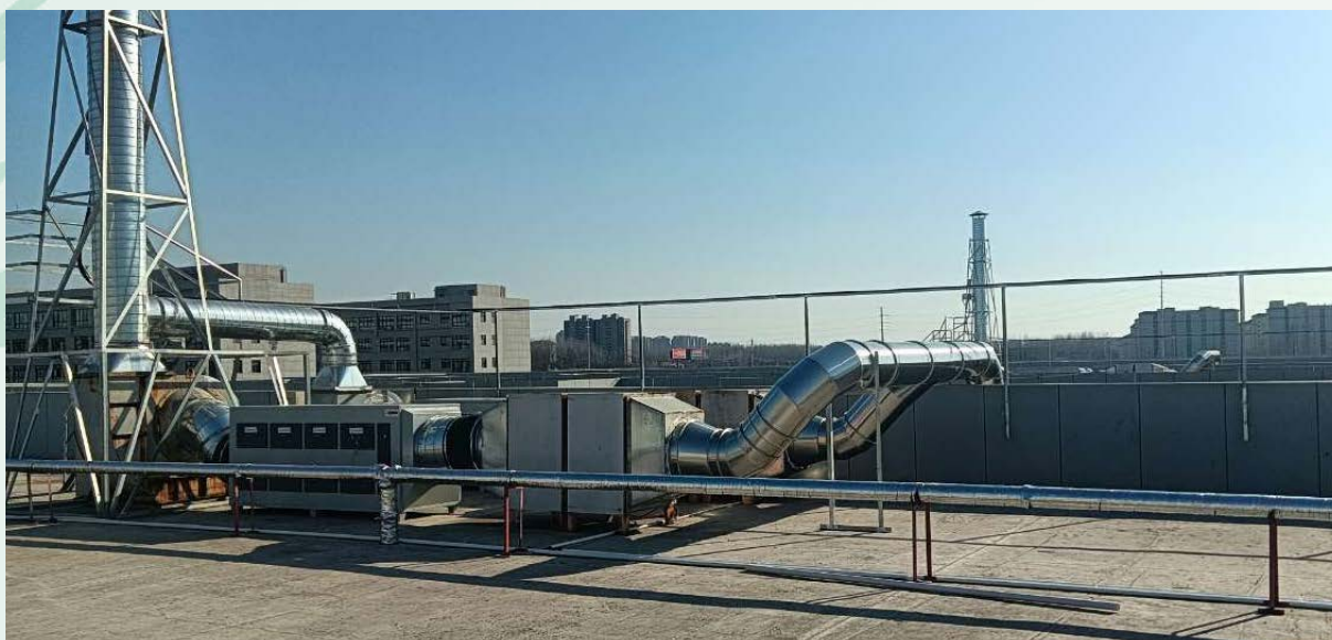
Activated carbon + photo-oxygen catalytic treatment equipment 活性炭+光氧催化處理設備
